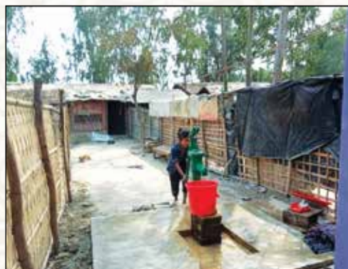
Water Points installed by DPHE at Ashrayan Community
